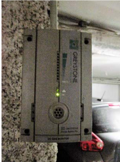
A wall-mounted Greystone carbon monoxide monitor activates the exhaust fan if a set level of CO emissions are detected.
