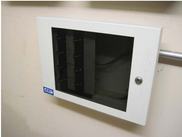
The alarm system also includes this smoke control panel which operates the stairwell pressurization and exhaust fans
