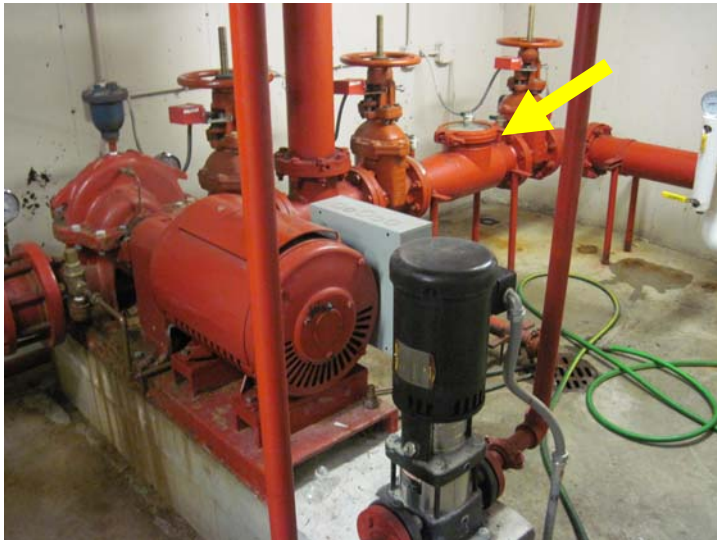
View of the building fire suppression system with 40-hp Lincoln electric AC motor, 1.5-hp jockey pump, and backflow preventer (arrow).
