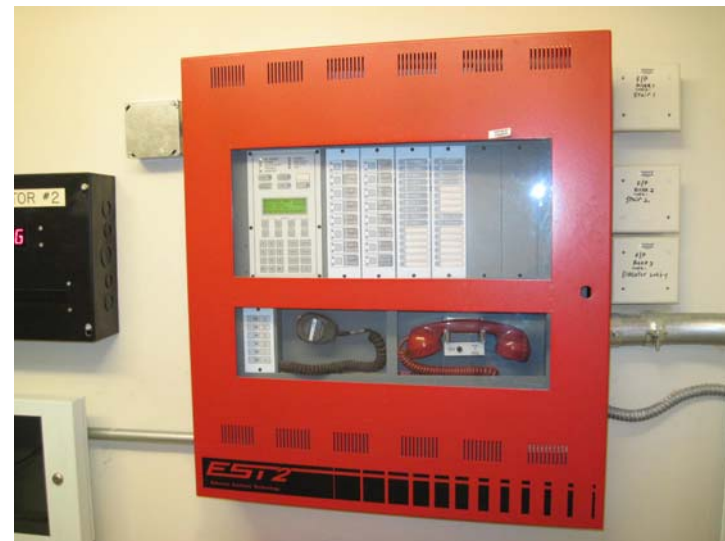
View of the Edwards EST2 fire alarm control panel with integrated command center, located in the entrance vestibule closet.
