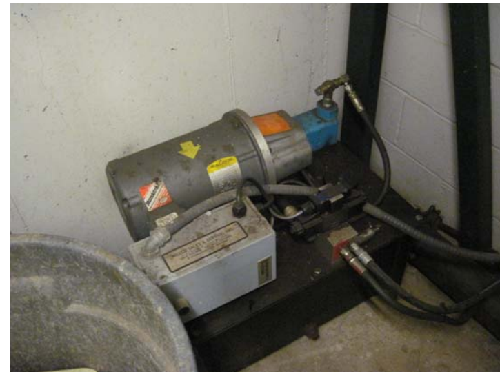
The compactor is operated by this Baldor 5-horsepower hydraulic pump.
