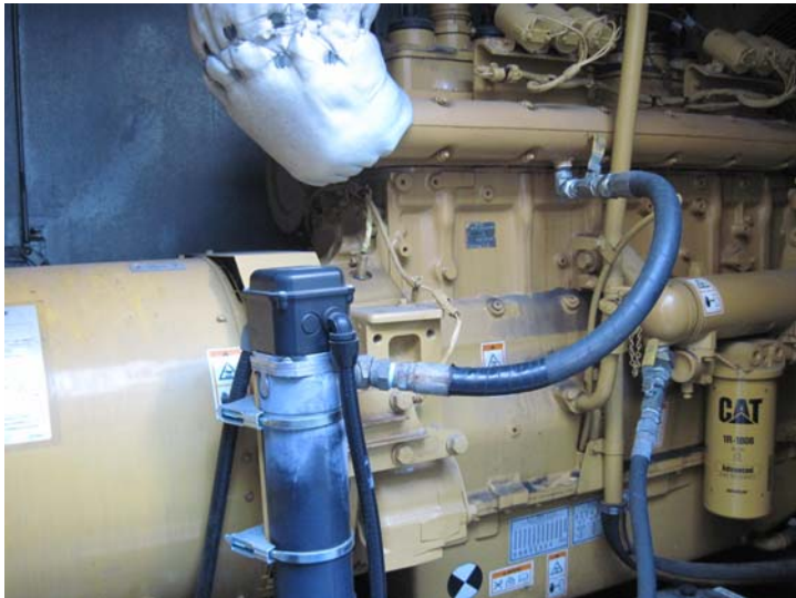
The rooftop Caterpillar 150 kW standby generator powers key building systems (elevator, fire alarm, lighting, exhaust fans) during a power outage.
