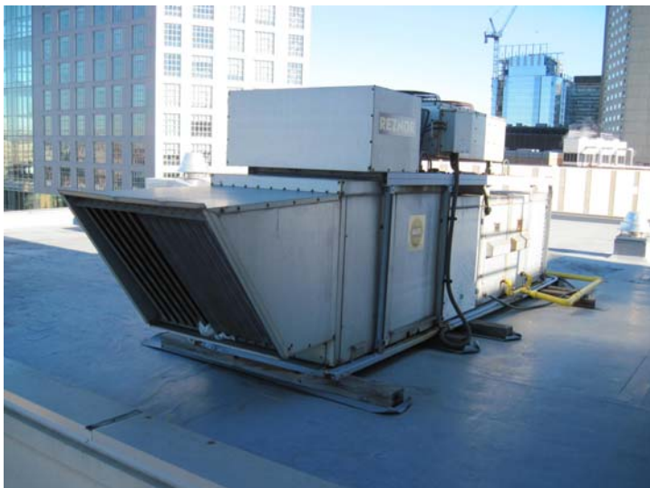
A Reznor makeup air unit (MAU) with 300-MBH gas heating unit and 22.5-ton electric packaged DX cooling unit provides fresh heated and conditioned air to the hallways and lobby.
