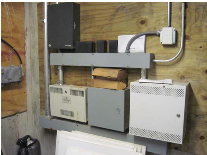
This Honeywell Pro-Watch 6000 secure entry access control system provides magnetic key-fob resident-only access to the building.
