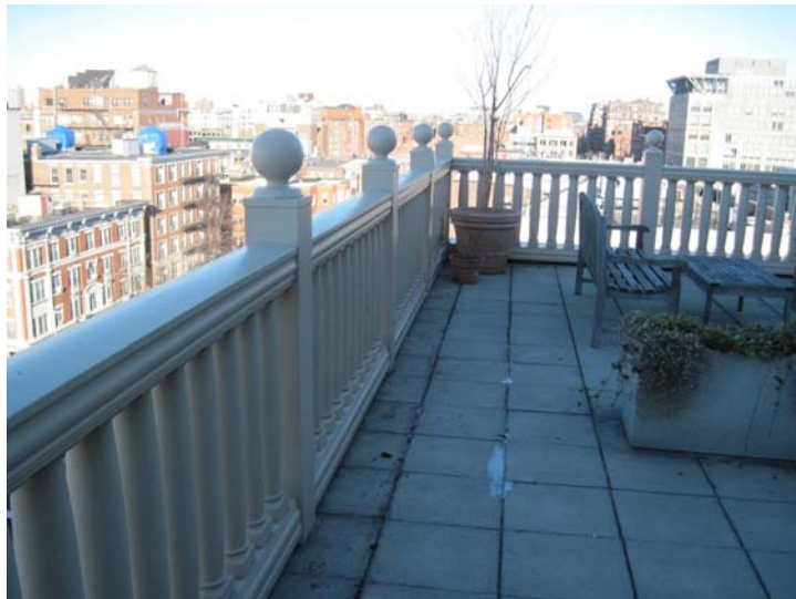
All terraces and balconies feature durable weather-resistant painted fiberglass reinforced plastic (FRP) railings and balustrades.
