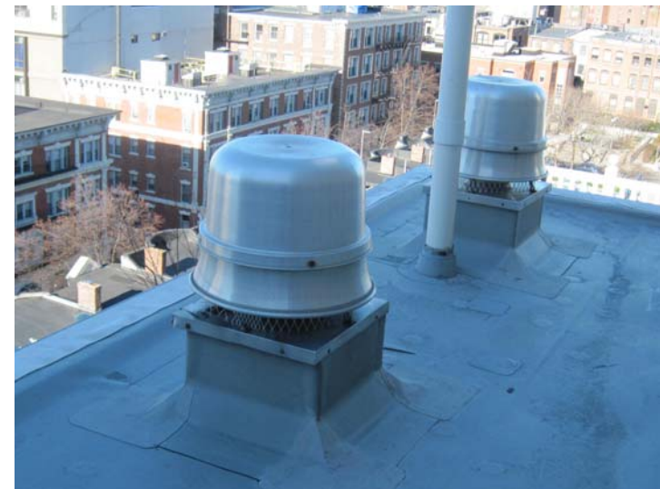
Several mushroom type rooftop powered fans serve the exhaust needs of the entry vestibule, trash room, and residence bathrooms, kitchens, and dryers.
