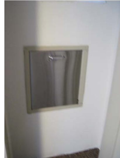
Each hallway feature a trash chute located in a closet at the north end of the hallway.
