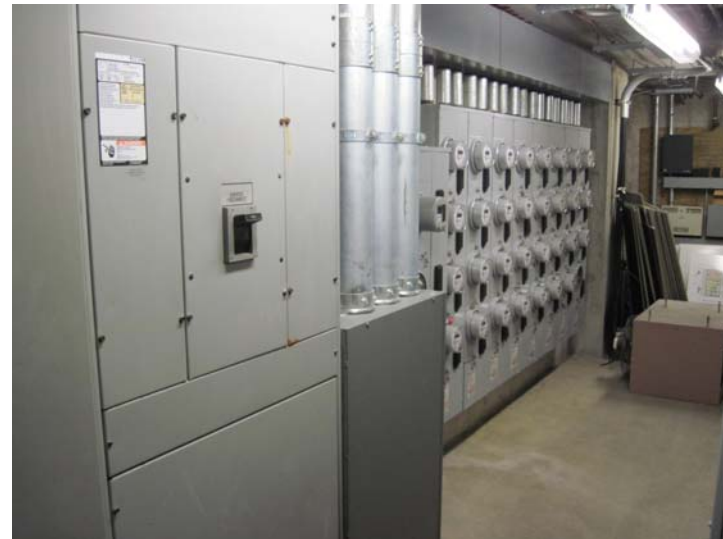
All residential units are individually metered for electricity usage
