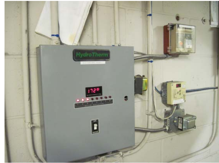
View of the HydroTherm boiler staging control panel (left) and HeatTimer outdoor temperature reset control (right).
