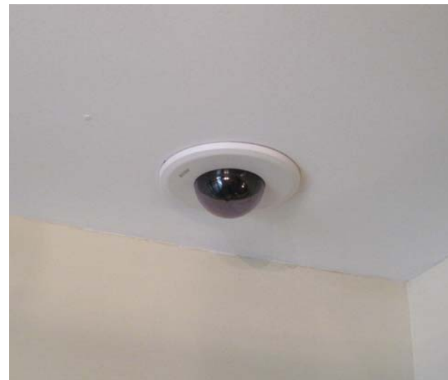
The building features a security system with statically placed interior and exterior mounted surveillance cameras.
