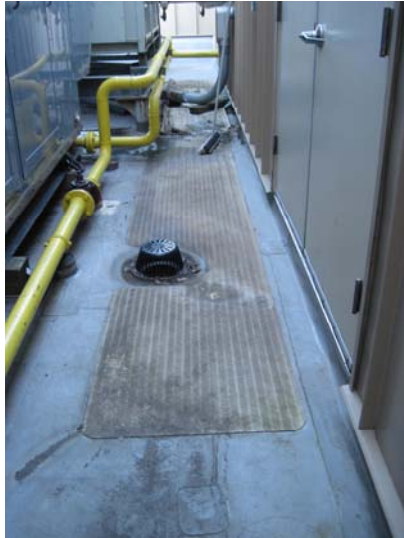
View of the lower roof TPO membrane located at the generator/chiller area outside of the 9 th Floor mechanical room.
