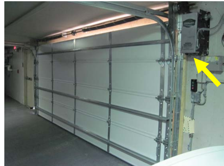
View of the newly replaced parking garage overhead door with wall-mounted LiftMaster power door opener (arrow).
