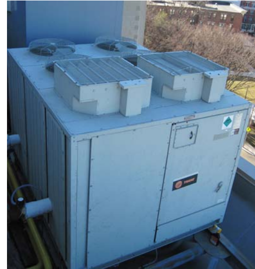
During the cooling months, the Trane 60-ton air-cooled liquid chiller removes heat extracted from the residences into the building loop via the fan coil units. The cooled building loop then cycles back through the fan coil units to extract more heat.
