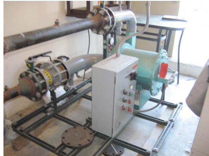
The building features an Eclipse centrifugal hermetic natural gas pressure booster system located at the 9 th floor common terrace storage room.
