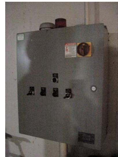
The garage features a double basin sand/oil separator system with dual 5-hp pumps and Weill 8151 duplex pump control panel designed to keep oil, sand, and other contaminants from entering the public sewer system.
