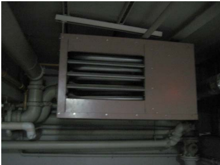
The parking garage is heated by two 100,000 BTU ceiling mounted Reznor FT100 natural gas fired horizontal unit heaters.
