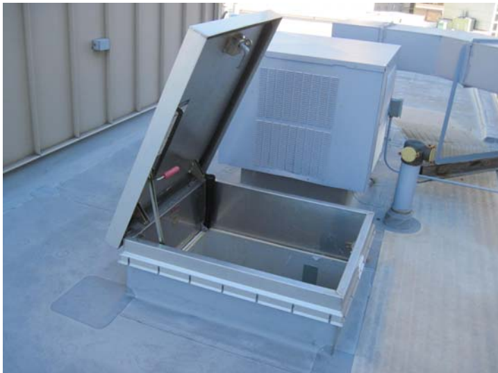
The roof is accessed via a metal spring-hinged roof access hatch located in the south stairwell.
