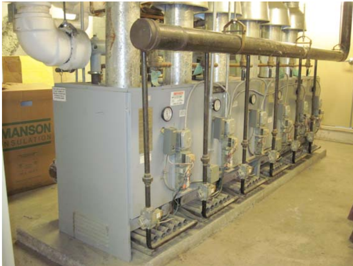
This HydroTherm Inferno Modular AG gas-fired hydronic boiler array (2,100 MBH input) serves the building resident unit heating needs via a 2-pipe system and unit-level vertical fan coil units (Whalen Units).
