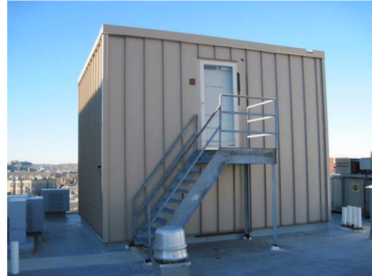
The elevator machine room penthouse features a durable standing seam metal cladding with galvanized steel access stairs.
