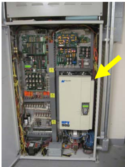
Both elevators feature solid state controls with Magnetek HPV-900 AC drives (arrow).
