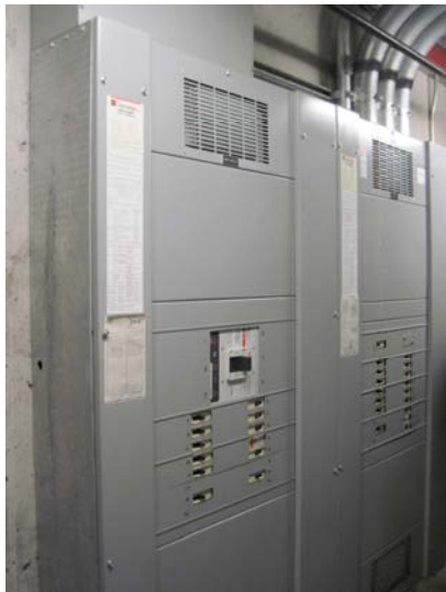
View of the Cutler Hammer building main disconnect panel
