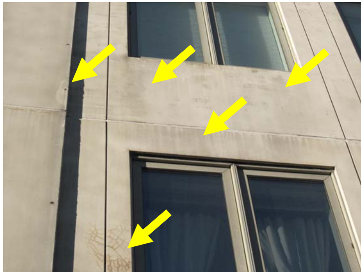
Close-up of localized spider-webbing and general overall surface deterioration of the GFRG cladding. (Viewed from front Mass Ave sidewalk looking at lower left corner of front building elevation)
