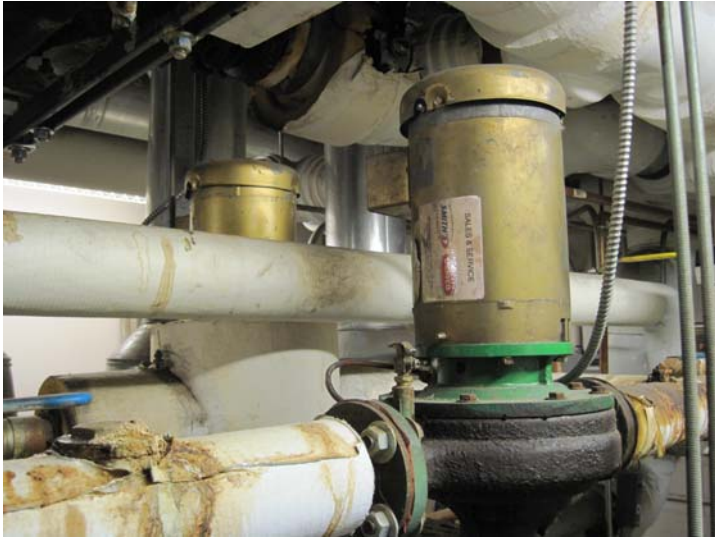
The domestic hot water is circulated by these Baldor 1.5-horsepower pumps. The primary pump runs continuously, and the backup pump is used only in the event that the primary pump fails.
