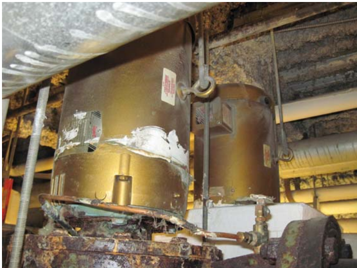
The main loop water is circulated by these Baldor 10-horsepower pumps. The primary pump runs continuously, and the backup pump is used only in the event that the primary pump fails.
