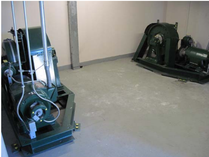
View of the two 20-horsepower elevator overhead traction machines located in the rooftop elevator machine room penthouse.
