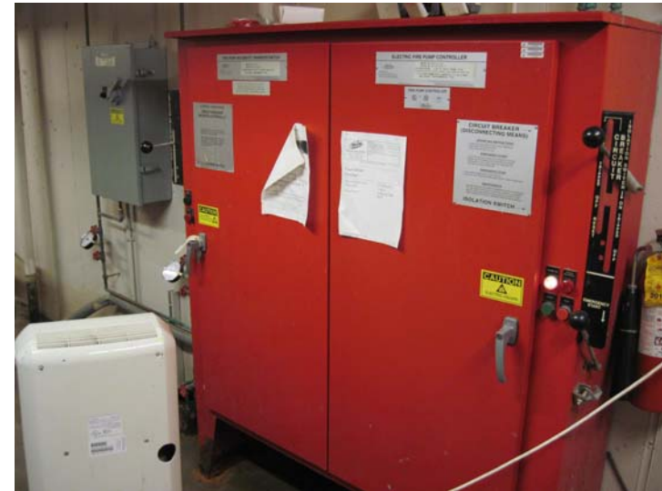
View of the Metron fire pump automatic transfer switch (left) and controller (right)
