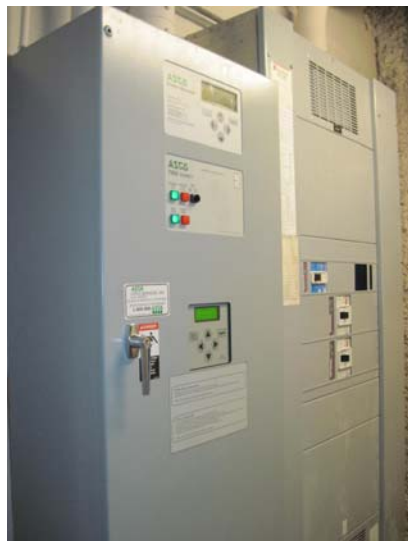
The ASCO 7000 series generator transfer switch is located in the adjacent rooftop boiler room.
