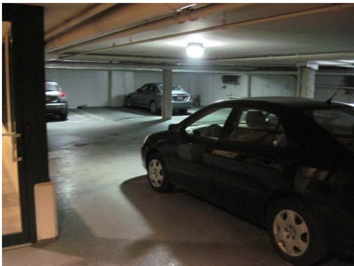
View of the sub-grade parking garage with ageing elastomeric traffic-bearing membrane
