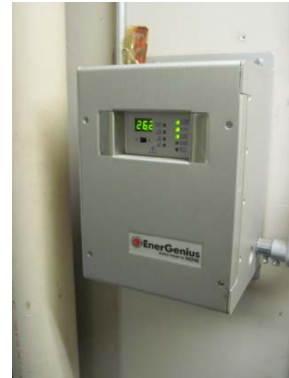
An EnerGenius generator engine-start battery charger located in the rooftop boiler room maintains the charge in the batteries that start the generator. An integrated battery fault alarm system detects battery problems.
