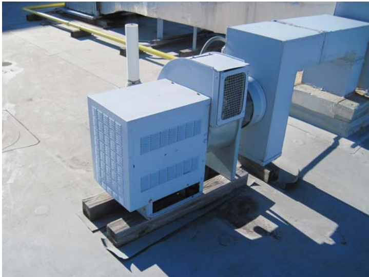
Three box-type stairwell and vestibule pressurization fans are activated by the fire alarm control panel during a smoke event to pressurize the stairwells and prevent smoke from entering the egress routes.
