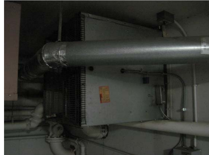
View of the CO detector and FACP controlled wall-mounted garage exhaust fan.
