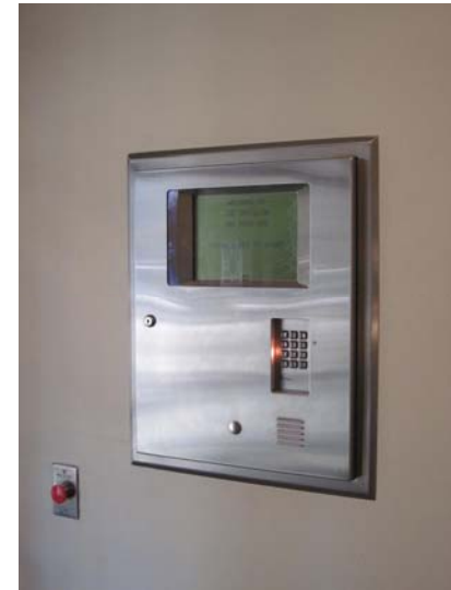
The wall-mounted phone-based entry intercom system provides remote controlled access into the building.
